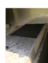
Clean air then goes through a fan (F6) and into the Treated Air Outlet (2) where it's released outside.
