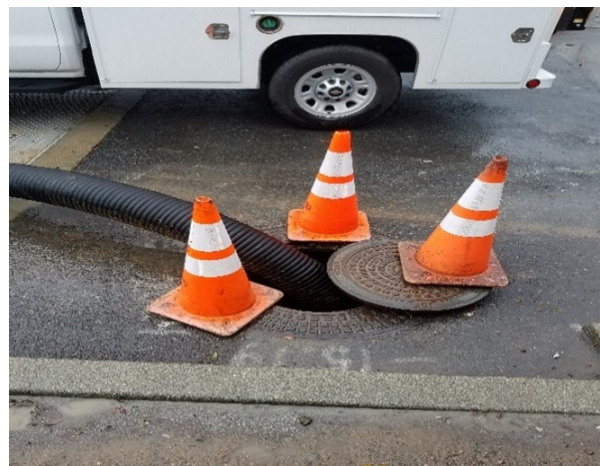
Bypass Pumping System
